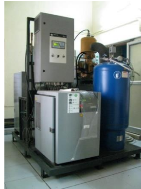
Liquid N 2 plant
