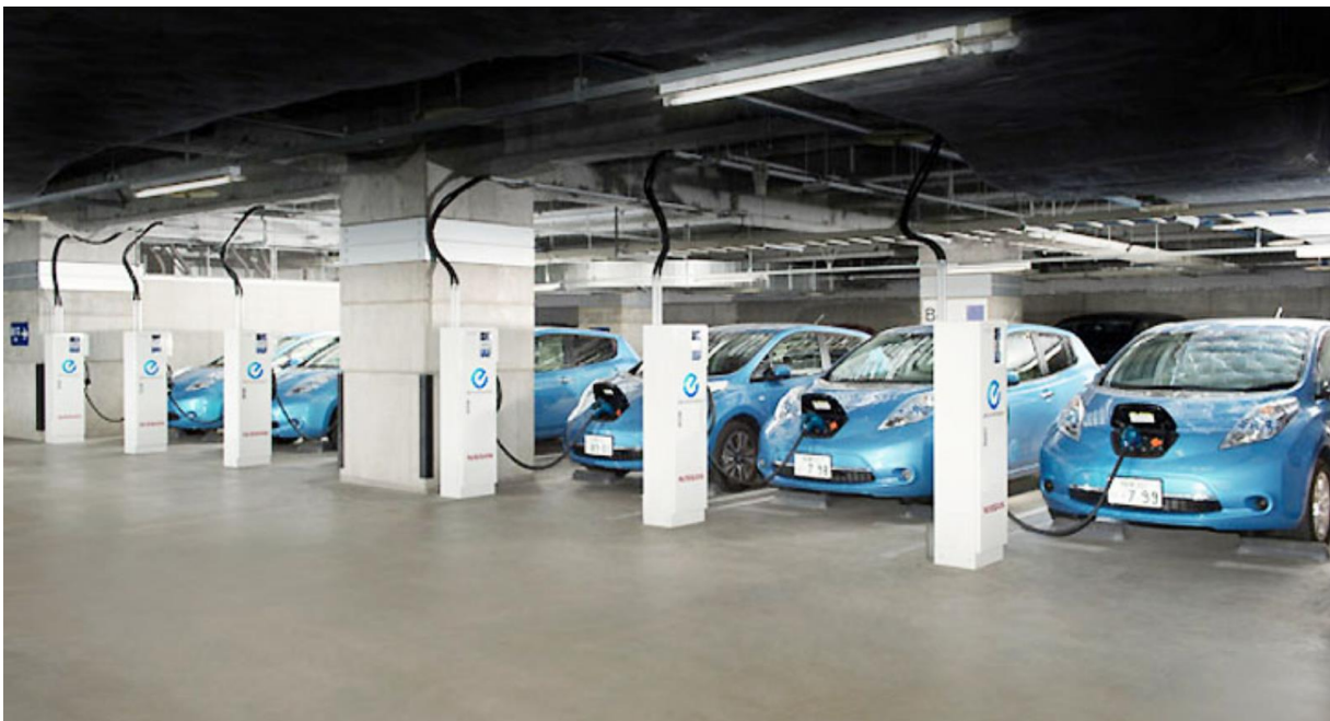
Figure 2:5 Fleet of Nissan Leafs being used as V2B resources to power an office in Japan 6
