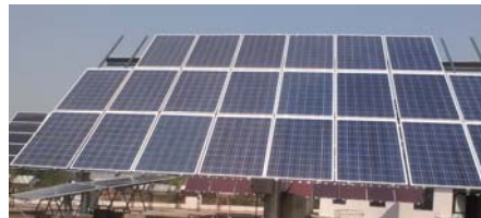
Multi-Crystalline Silicon modules on 2D Tracker installed at SERE
