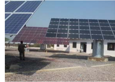
Thin Film Amorphous Silicon and CIGS modules on 2D Tracker installed at SERE
