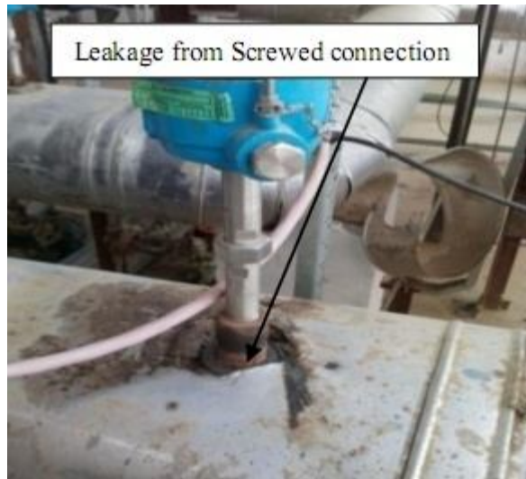
Fig 36: Temperature transmitters leakages
