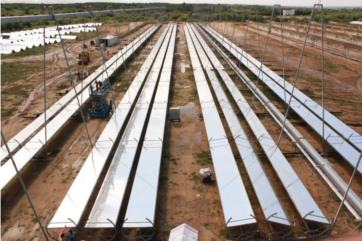
Fig 4: The LFR field installed at site.
