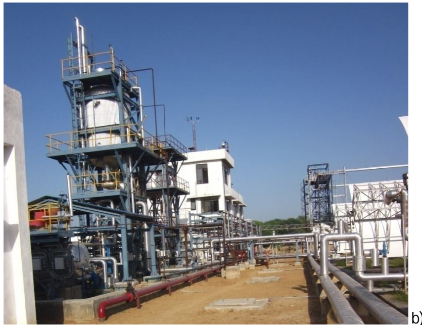
Fig 11: a) The under construction Building along with other support structures. b) The completed structures.
