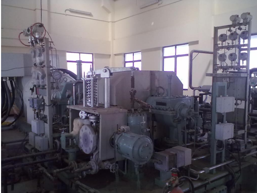
Fig 7: Steam Turbine system with accessories
