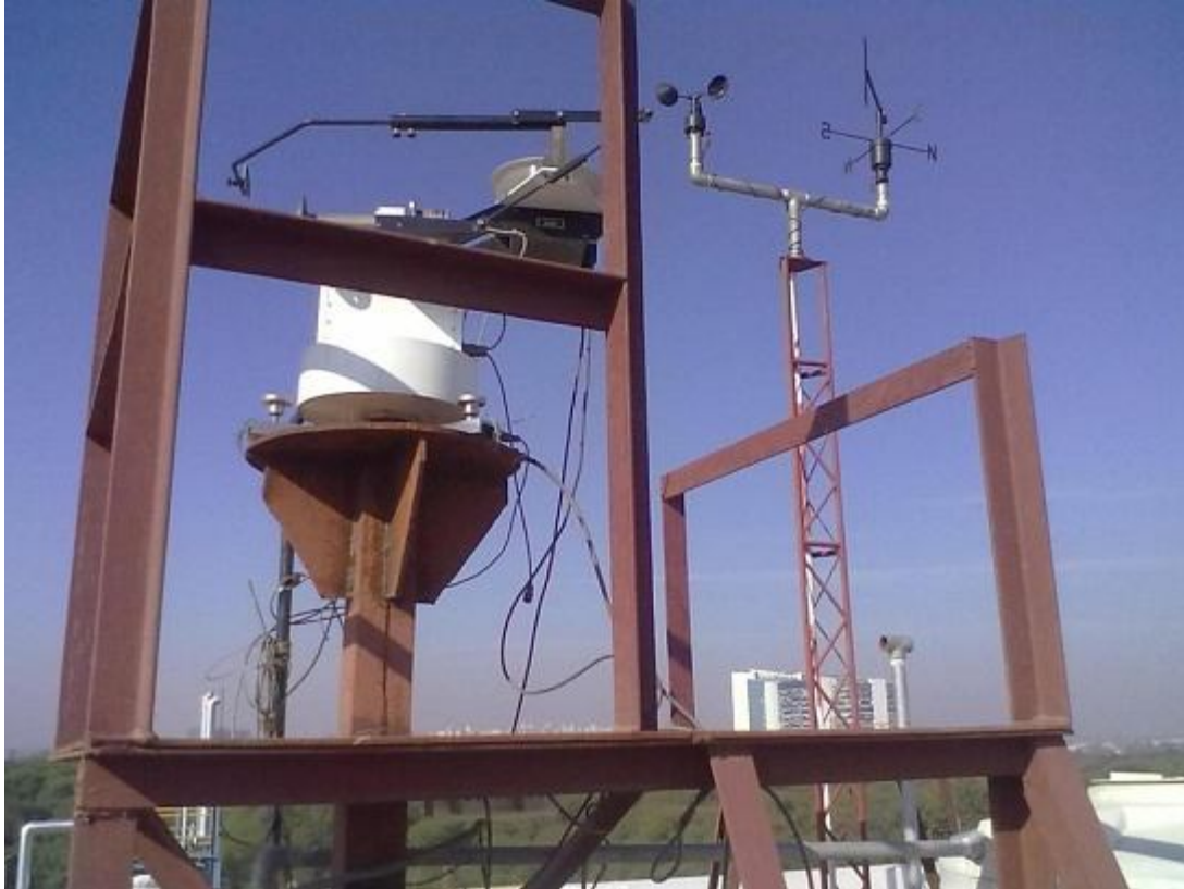
Fig 10: Whether station installed at site
