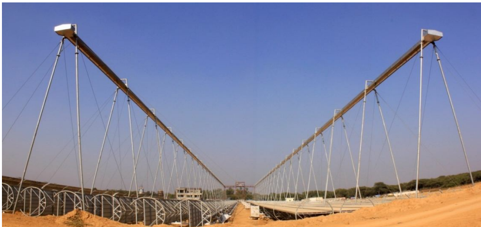
Fig 26: Linear Fresnel Reflector Solar field
