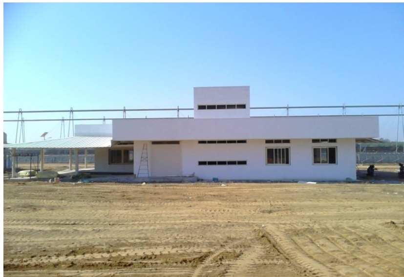
Fig 15: The Test Facility control building
