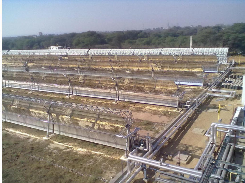
Fig 25: The Parabolic Trough Solar Field.
